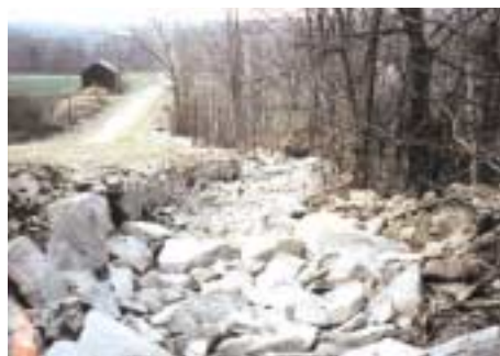
Road ditches are a sediment-producing threat in this hilly region. The USC is installing various practices to reduce this problem.
