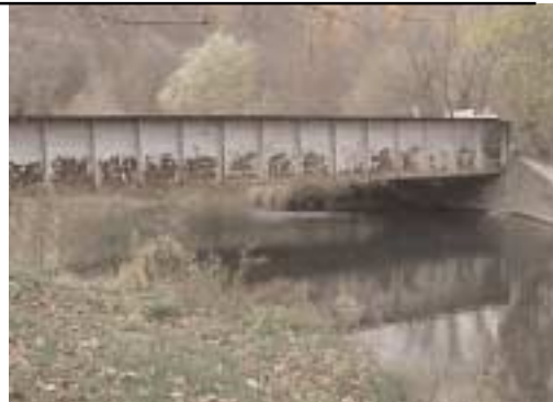
In a unique floodplain enhancement project, Chemung County will remove this bridge which collects debris and dams the creek during high water periods.
