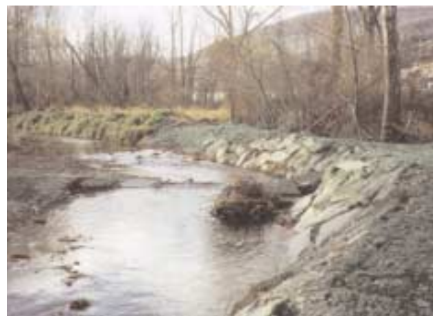
A rock weir, root wad and rip-rap in Cold Brook in Steuben County depict some of the old and new technologies available for stream restoration.
